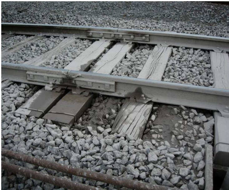
Mud pumping zone
